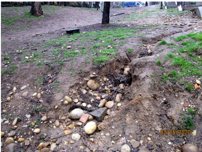
Deep erosion in the park at 19th and Lamont
